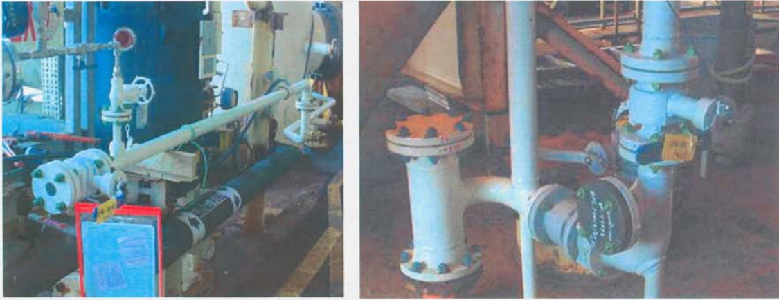
Figure 3 - Typical 'Cut-ins' Offshore Work Pack Piping Installations
