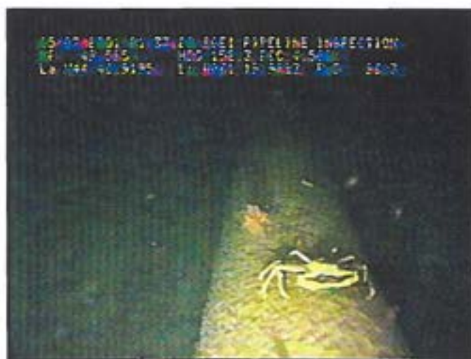
Photo 18 Snow Crab on the Main Pipeline
