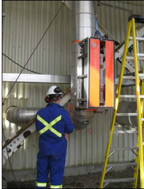
BCT Scanner on Insulated Piping
