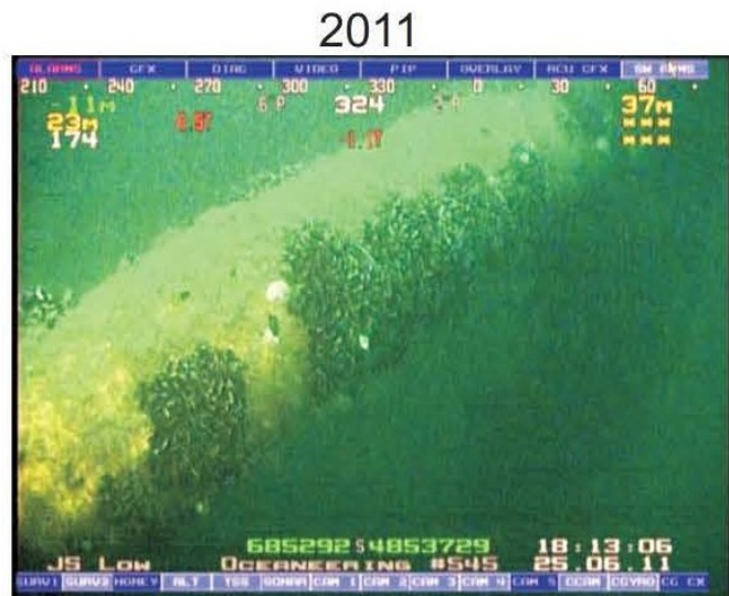
Moderate marine growth on East horizontal brackets at WHPS M-79A in the 2011 survey.
