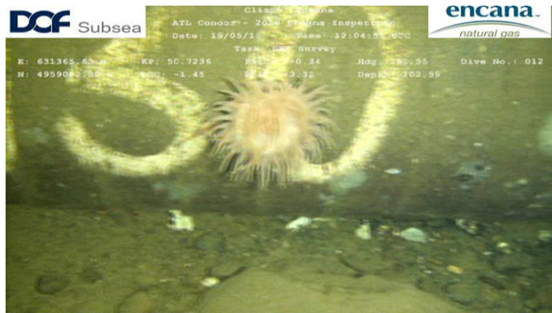
Tube anemone affixed to side of pipeline at KP 50.72
