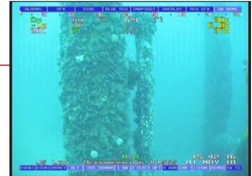
Heavy marine coverage of hydroids on the AN-06 anode.
