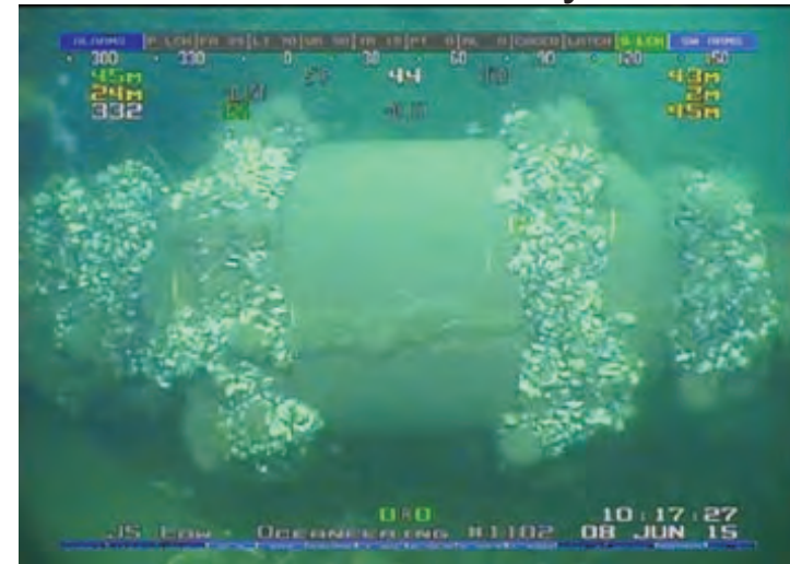
Similar mussel growth to 2013, with additional hydroids. Possible hydroid colonization along the horizontal seam of the insulation cover. (2014 photo not good quality to compare).
