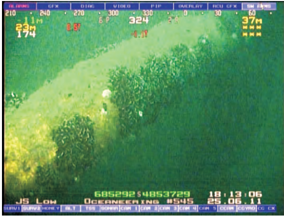
Moderate marine growth on East horizontal brackets at WHPS M-79A in the 2011 survey.
