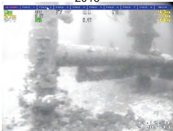
Similar sparse marine growth at the base of a leg of WHPS D-41. Possible cleaning may have taken place.
