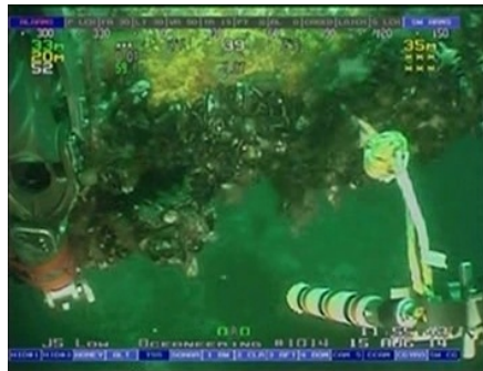
Dense mussels on the south crossbar between Legs 3 and 4
