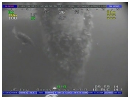
Hydroids and mussels cover the middle of Leg 4. A cunner is visible swimming near the structure.
