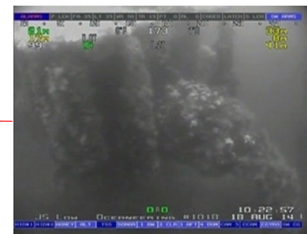
The subsea tree inside the wellhead protection structure, covered with mussel, sea star and frilled anemones
