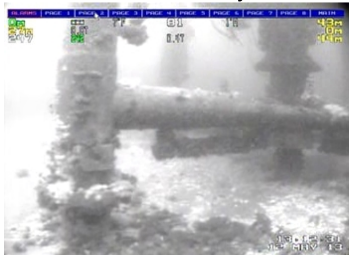
Similar sparse marine growth at the base of a leg of WHPS D-41. Possible cleaning may have taken place as evidence by the organisms on the surrounding sea floor.
