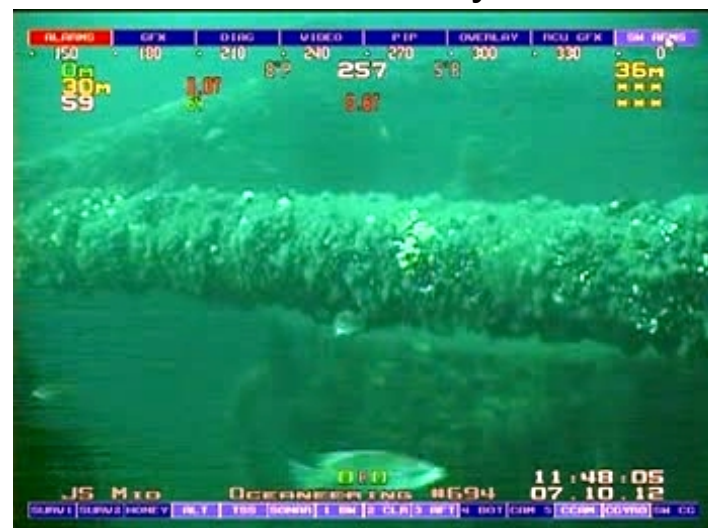
Significant growth of marine fauna on East horizontal bracket at WHPS M-79A in 2012
